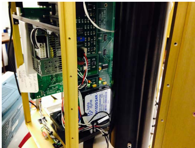
Figure 10: MPS-2 power distribution board. Notice green LED's indicate good power levels.
