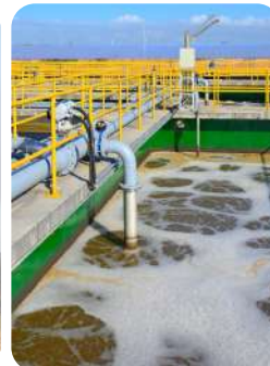
Industrial facilities with water treatment
