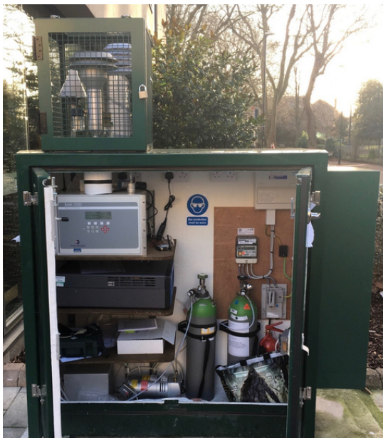
Figure 1: An ET PR5 Professional Air Quality Monitoring Station
